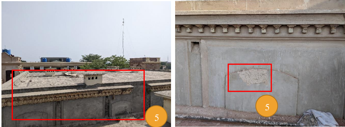
Figure 8. Cement Destroying Walls and its Elements
