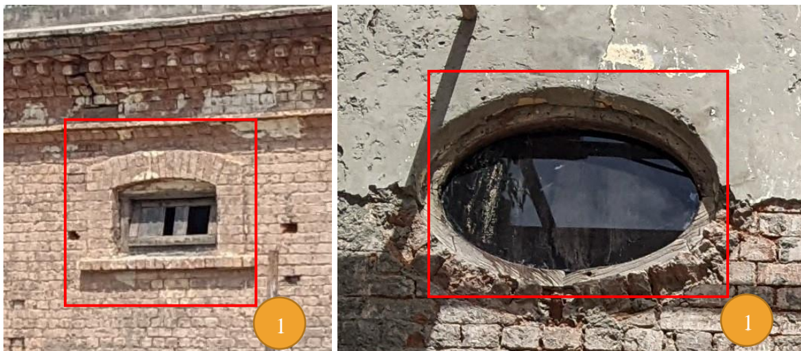
Figure 13. Condition of Ventilators
