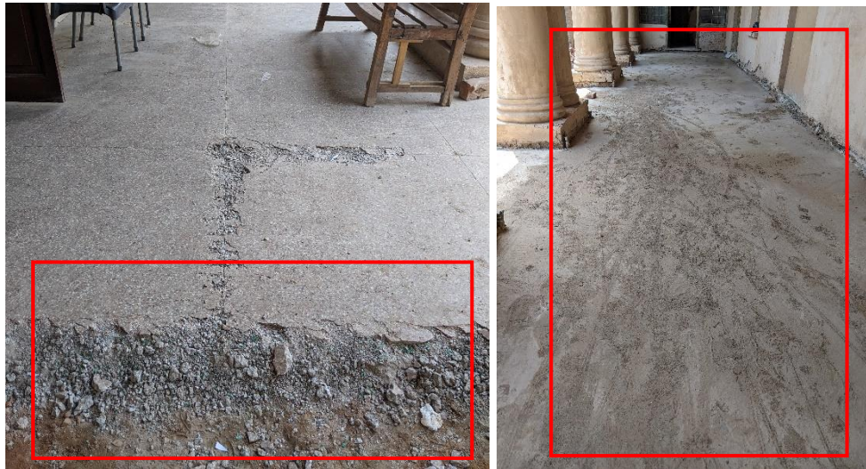
Figure 12. Condition of Floor
